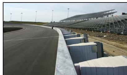
The entire outside wall at Iowa Speedway is comprised of the SAFER Barrier system.
